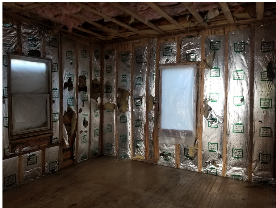
Photo 6. Final clearance photo of Rutherford House interior following removal of sheetrock wall and ceiling materials.
