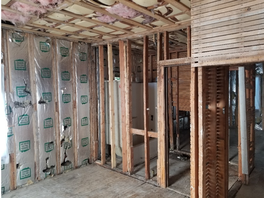
Photo 5. Final clearance photo of Rutherford House interior following removal of sheetrock wall and ceiling materials.
