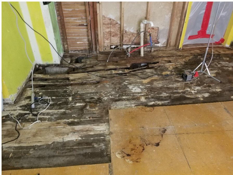
Photo 8. Water damaged subfloor materials in the Comes at Night House kitchen. Owner will be responsible for removal of moldy wood subfloor.
